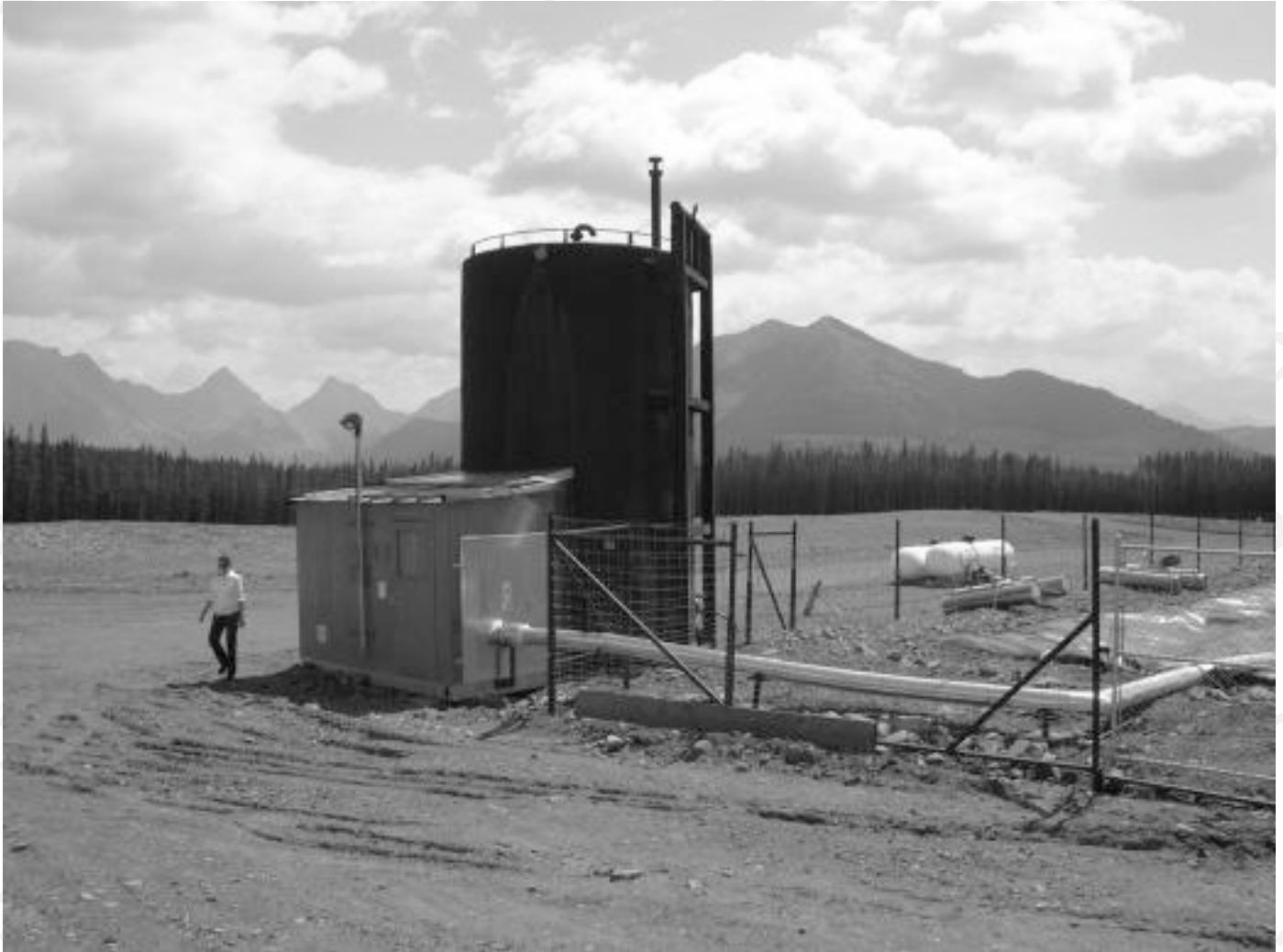
Coalbed methane gas wellhead
